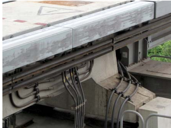
Figure 5: Auxiliary power pick up rails
