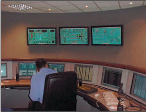
Figure 8. Unit 1 control desk with the new LOMIS systems installed
