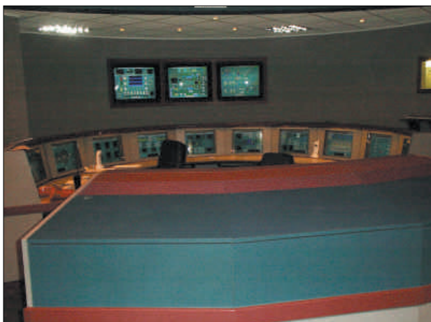
Figure 7. Unit 3 control desk with LOMIS installed (Courtesy of ScottishPower)
