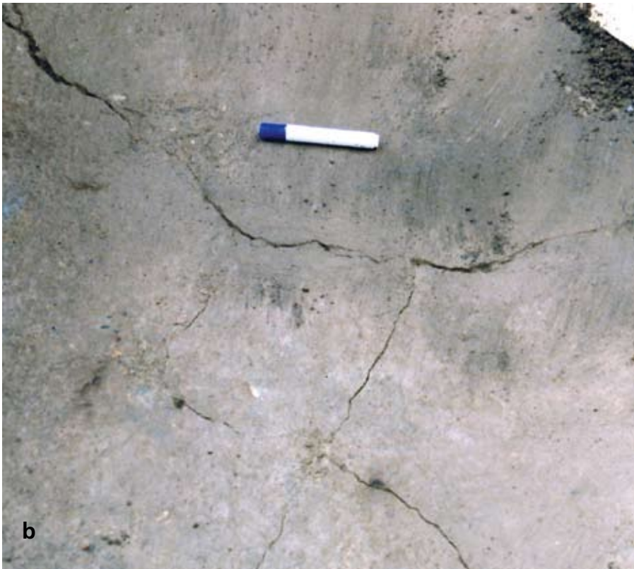
(b) Map pattern cracks in sulfate-attacked oversite concrete beneath a suspended wooden floor of an adjacent room.
