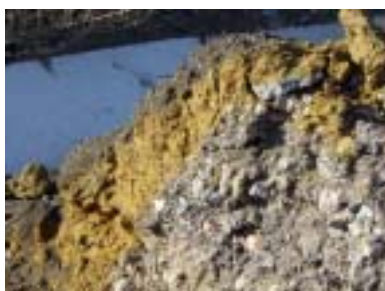
Figure 7.3 Photo taken from of a road widening scheme, showing the cross section of a slope composed of sub-base consisting of recycled material, covered with sub-soil and a layer of top soil for vegetation growth.
