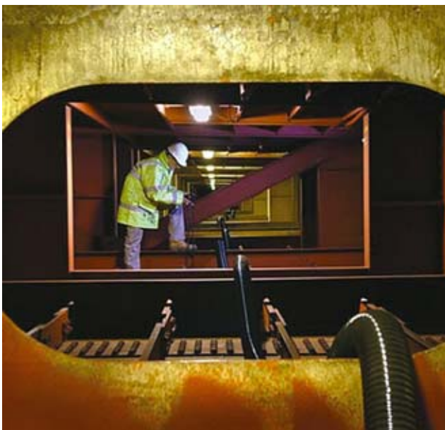
Using tried and tested techniques to deliver cost effective engineering solutions – M1 Tinsley Viaduct
