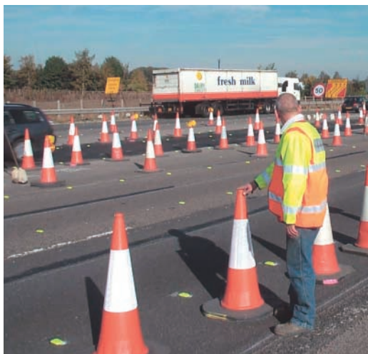
Hard hats are not worn by TM operatives who are working adjacent to the live carriageway. Hard hats are compulsory in all other cases.
