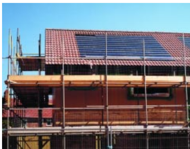
Installing the counter battening to provide an air gap for cooling behind the tiles
