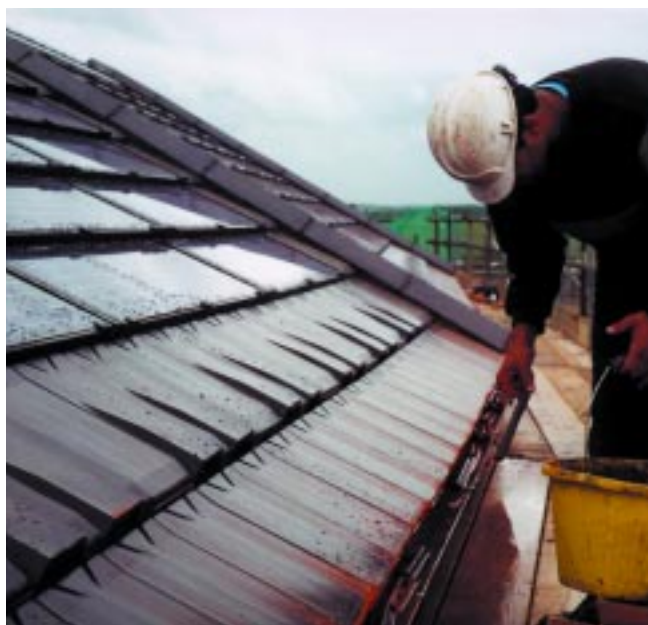
Final touches to the roof, showing the PV, ventilation tiles and ordinary tiles cut to fit at their lower edges
