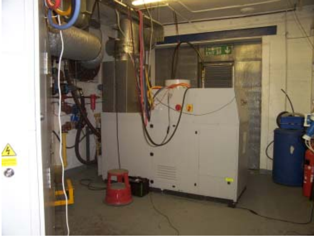
Figure 5.3.1: Bowman Power's TG50 on test
