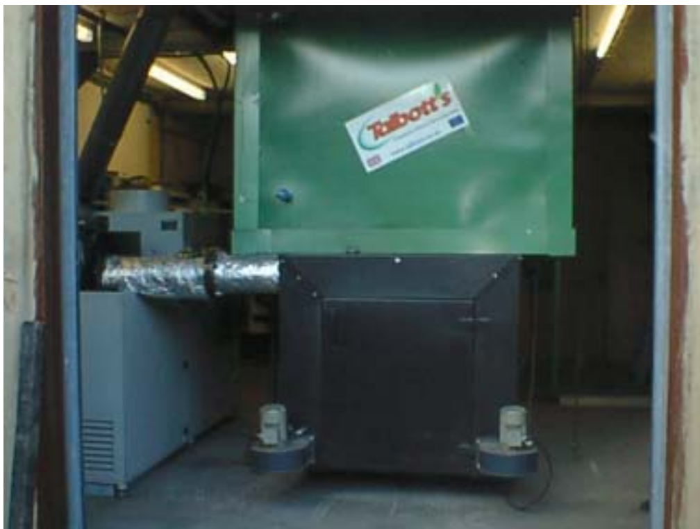
Figure 3.2.1: Biomass Combustor connected to Micro-Turbine
