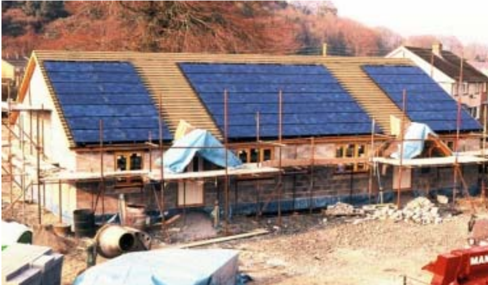
Fig. 2: The bungalows showing gap in PV array above entrances (BRE).
