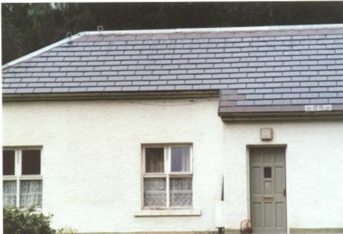
Fig.9: Typical PV roof on Glen Lyon site (BRE).
