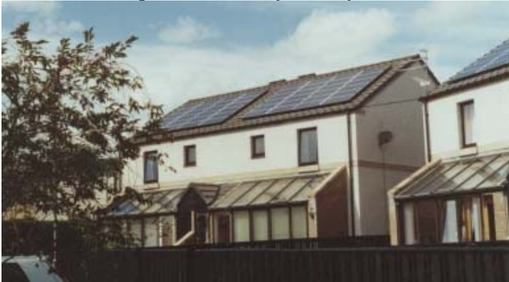
Fig.15: Retrofit PV arrays at Coldstram (BRE)
