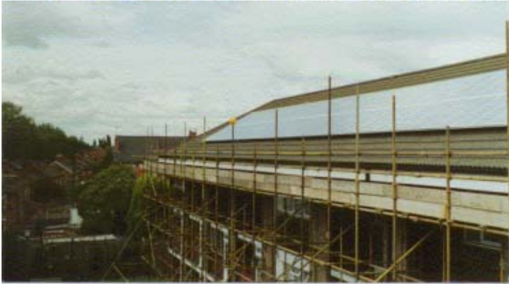
Fig.13: Rear view showing PV roof (BRE)
