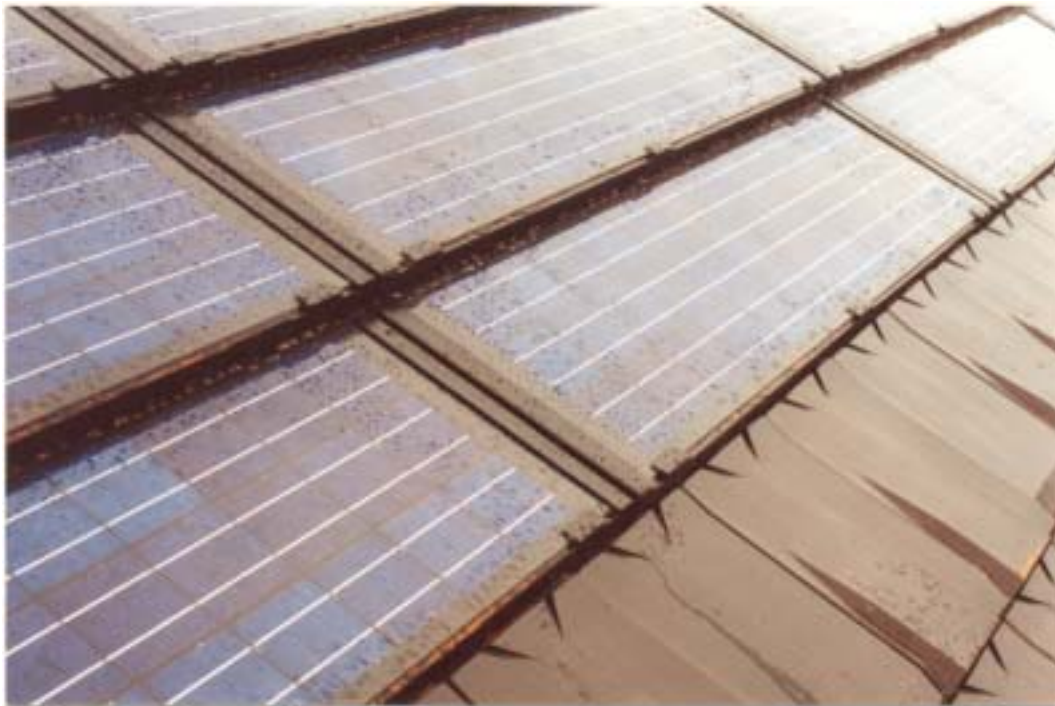
Fig.8: Close up Pfleiderer Terra Piatta solar tiles and vent tiles below (BRE).
