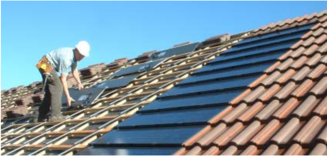
Fig. 5: The Redland roof integrated PV system (BRE).
