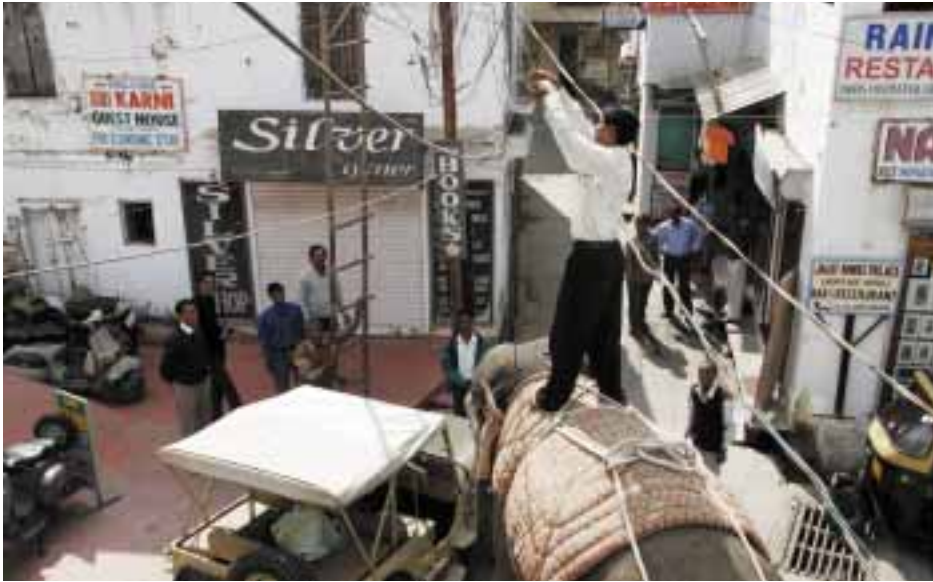
Traditional and modern: fixing wiring in Rajasthan, India. QILAI SHEN | PANOS PICTURES
