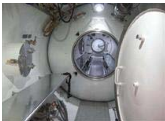
A view of the treatment chamber looking through to the 30-person main decompression chamber
