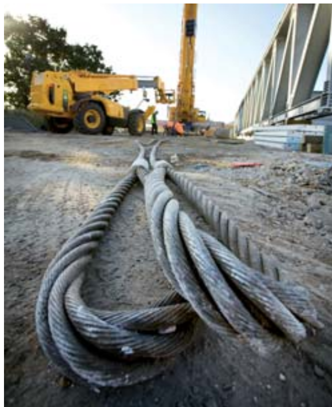
Steel hoists for lifting temporary bridge across the River Lee into place
