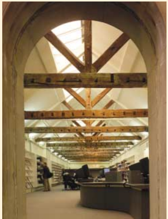
King Charles Court: removal of modern casings and partitions has allowed the display of the historic trusses in the new library for Trinity College of Music.
