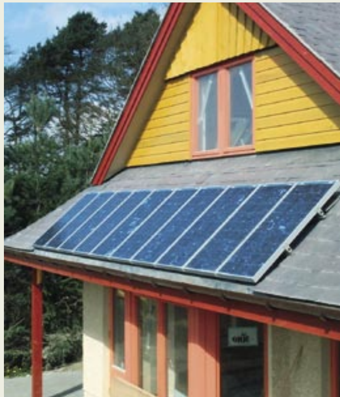
Camphill, Aberdeenshire – solar photovoltaic installation part-funded by DTI Major Demonstration Programme.
