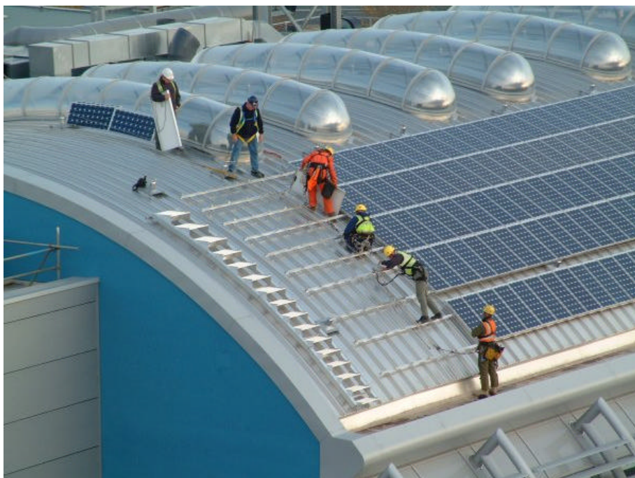
Installing photovoltaic panels on Newcastle University's new, six-storey flagship Devonshire building. Home to the Environmental and E-science Research Centre, the design of the steel-framed building incorporates many sustainable design features and is the first University laboratory in the country to achieve the BREEAM 'Excellent' rating.
